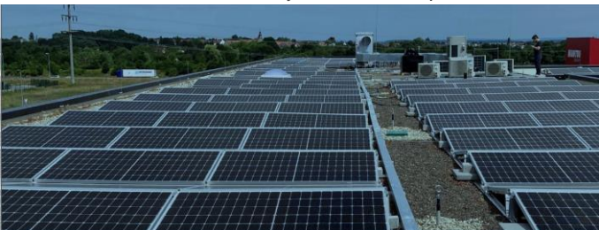
Photovoltaic system at axicorp in Friedrichsdorf
