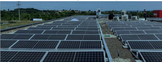
Photovoltaic system at axicorp in Friedrichsdorf
