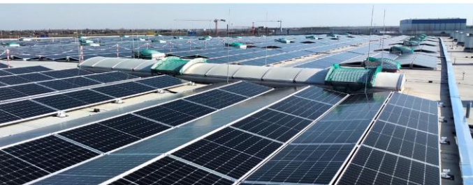
Photovoltaic system at the main production site of mibe GmbH Arzneimittel in Brehna
