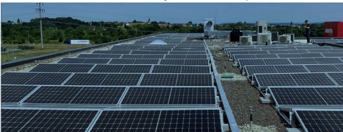
Photovoltaic system at axicorp in Friedrichsdorf
