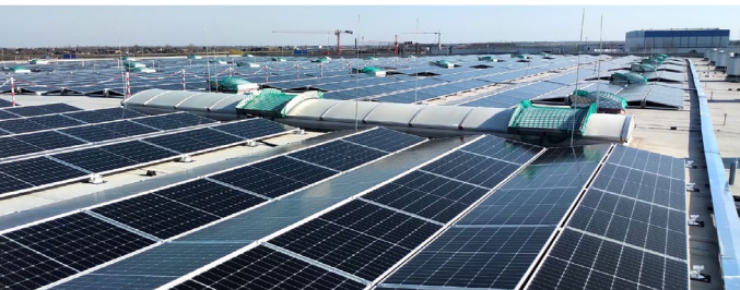
Photovoltaic system at the main production site of mibe GmbH Arzneimittel in Brehna
